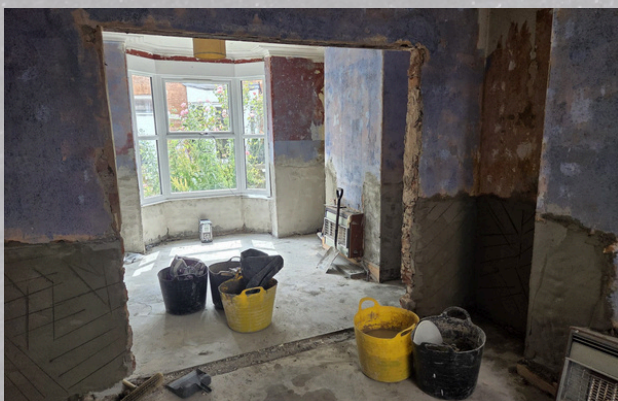
Reception Rooms (Damp Works)
